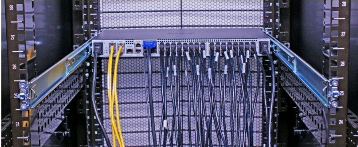
Figure 4: Four Post Rack: System and Cables Installed
