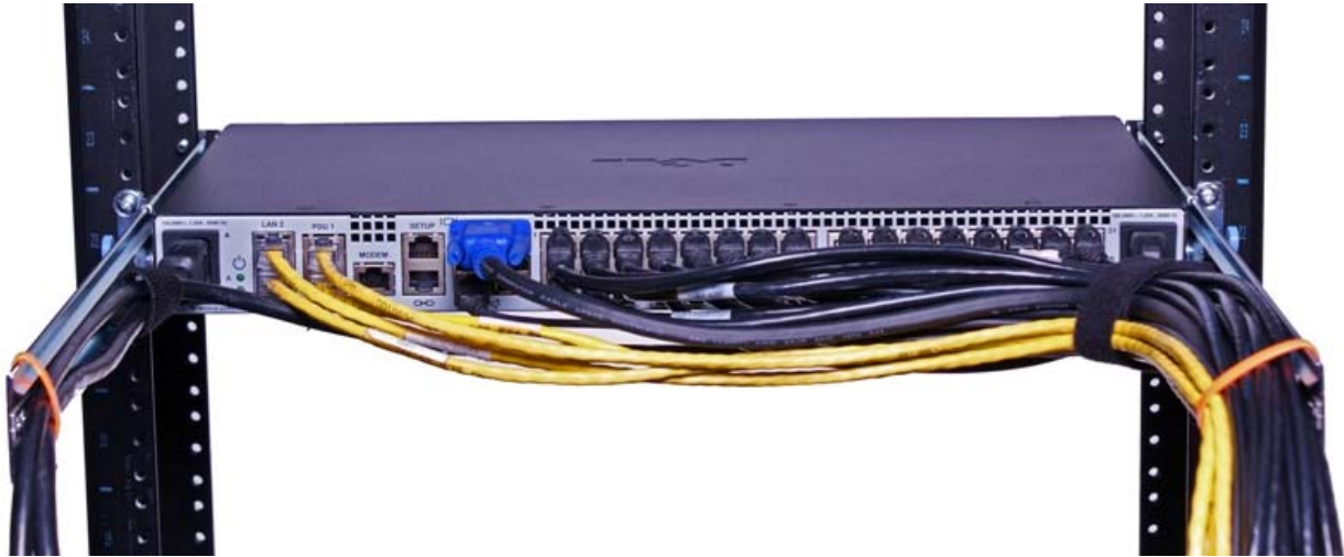
Figure 9: Two Post Rack: Routing Power and Data Cables (Optional Tie)
